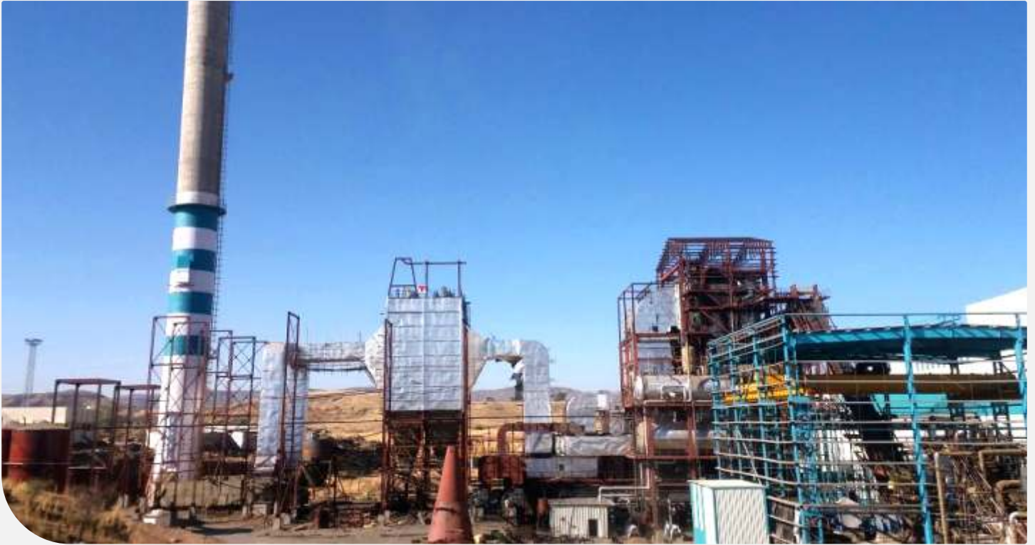
Sharayu Agro Industries Ltd. 160 TPH, 87 Bar, 520°C
